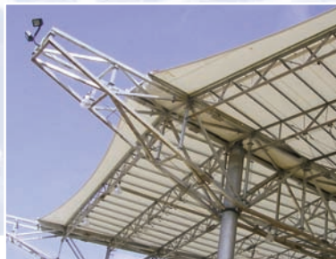
During Deployment, the 8028 was anchored after tensioning. The designers utilized product mechanical characteristics to maintain a fully tensioned roof upon completion.
